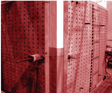
Pins and centerhole jacks are installed on two of the tower skins in order to complete the phase 1 bolting of the connection; further allowing the rigging to be disconnected from the top of the tower lift
