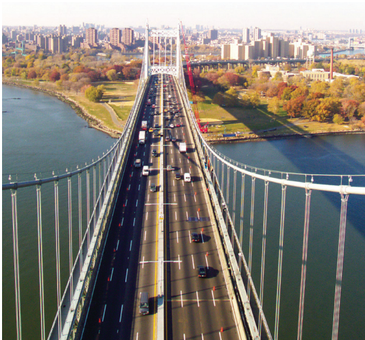
AB performs structural improvements to the RFK Bridge during live traffic; the bridge carries 150,000 vehicles daily
